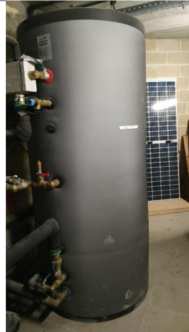
Figure 3. DHW – Aerothermal System
